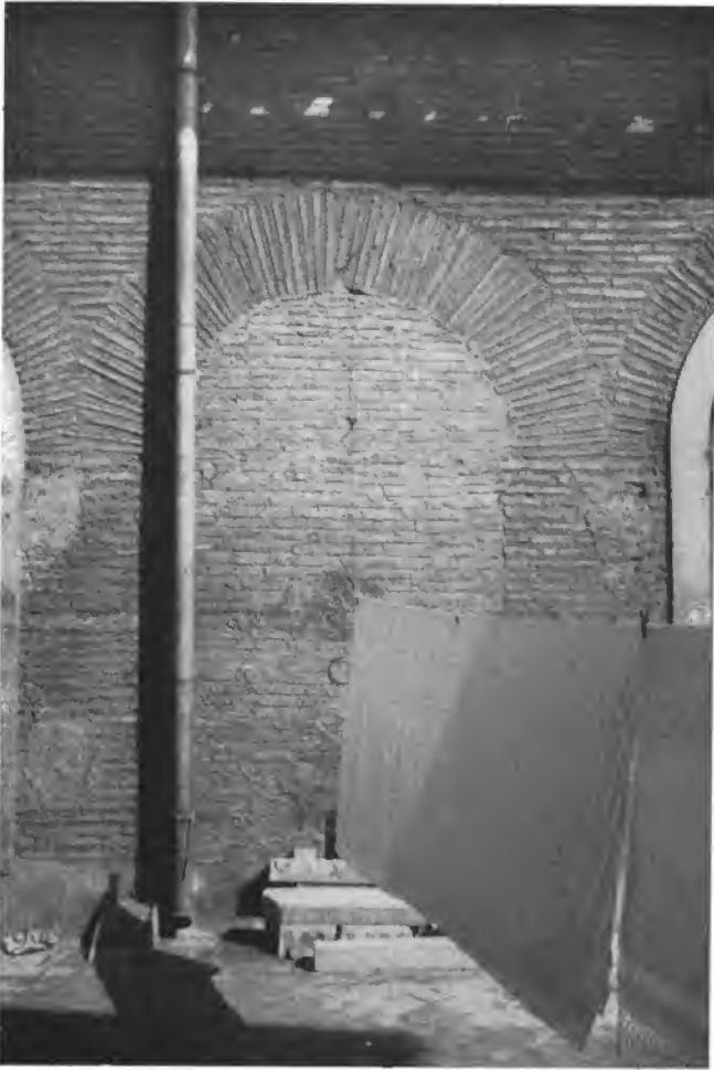
Fig. 44a. S. Maria Maggiore, South flank, sixth window with thirteenth century blocking
